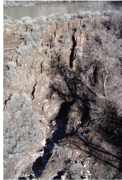
Figure 3-15. Schroeder Dam in Beaver Dam State Park. Erosion cut into the front face of the earthen dam.
